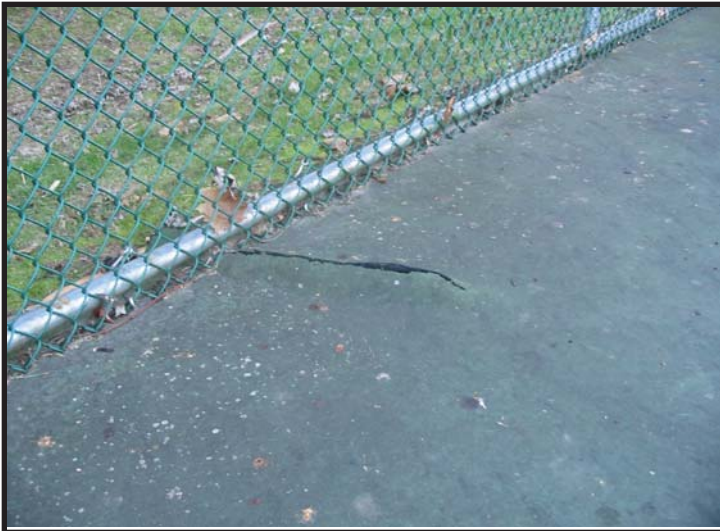
Bamboo beginning to shoot up through tennis court at Lewis Park causing damage
