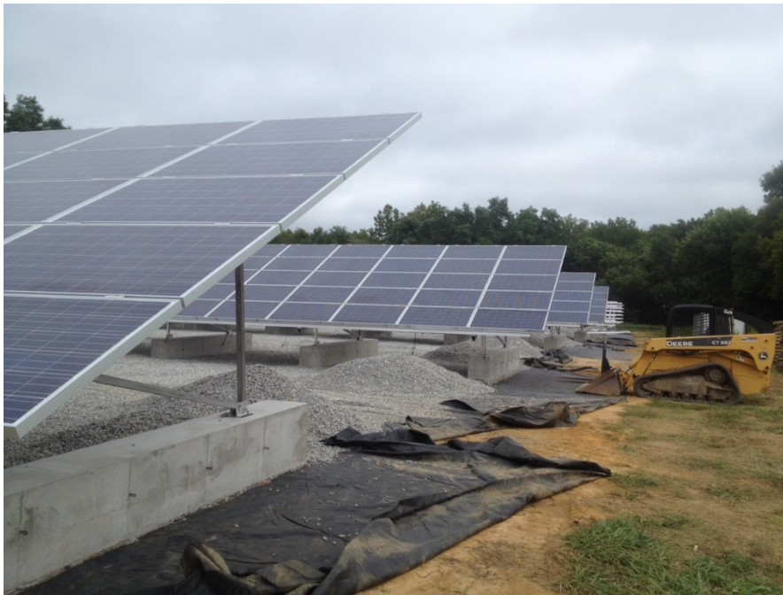
Figure 1: Solar Panels installed at McKees Park
