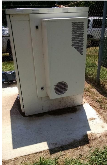
Figure 7: Fiber Distribution Cabinet
