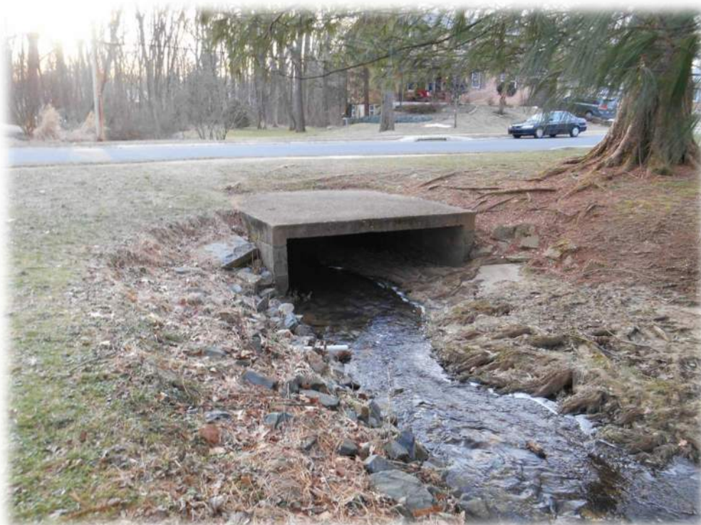
Figure 3 – Upstream Box Culvert Opening (Note root growth into the culvert)
