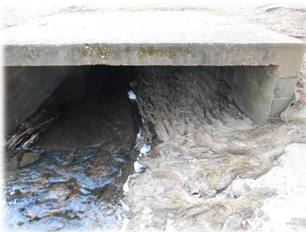
Figure 4 – Root Growth into Culvert
