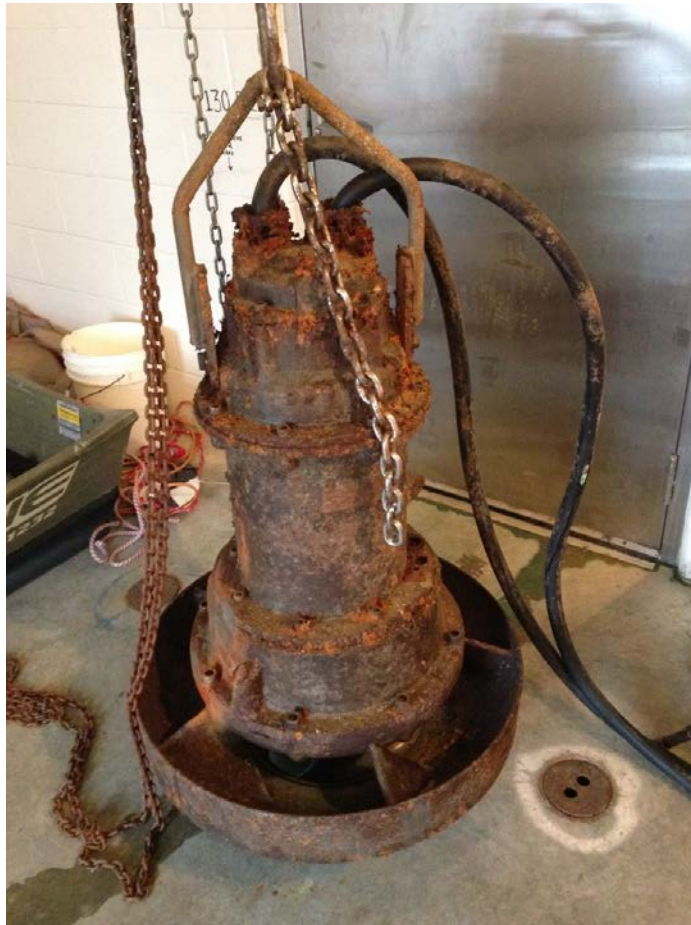
Reservoir I/O Tower Pump with wear at the cable connection
