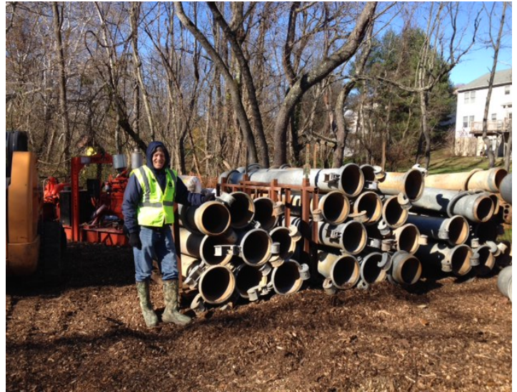
Steve Williams, DNREC, with piping used to pump creek flows around the work site.
