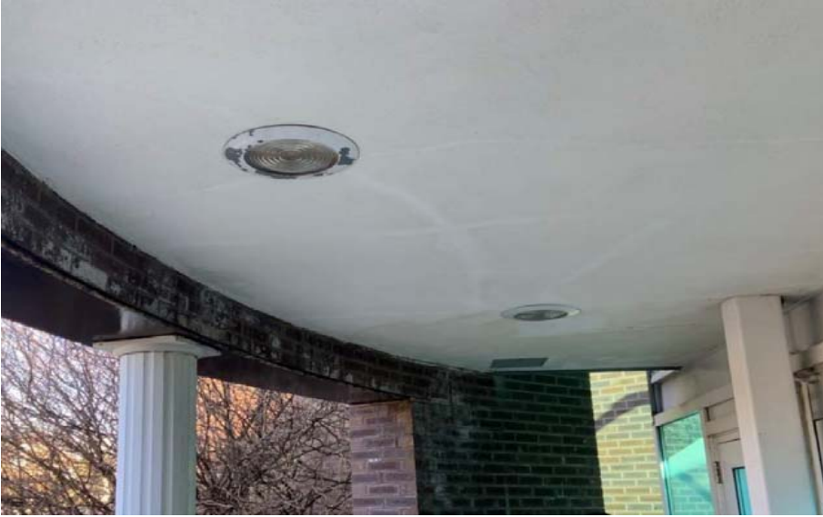
Image #7: Typical lentil and efflorescence in brick. Note condition of ceiling showing water damage.
