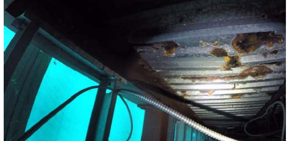
Image #2: Typical steel decking holes and buckling.
