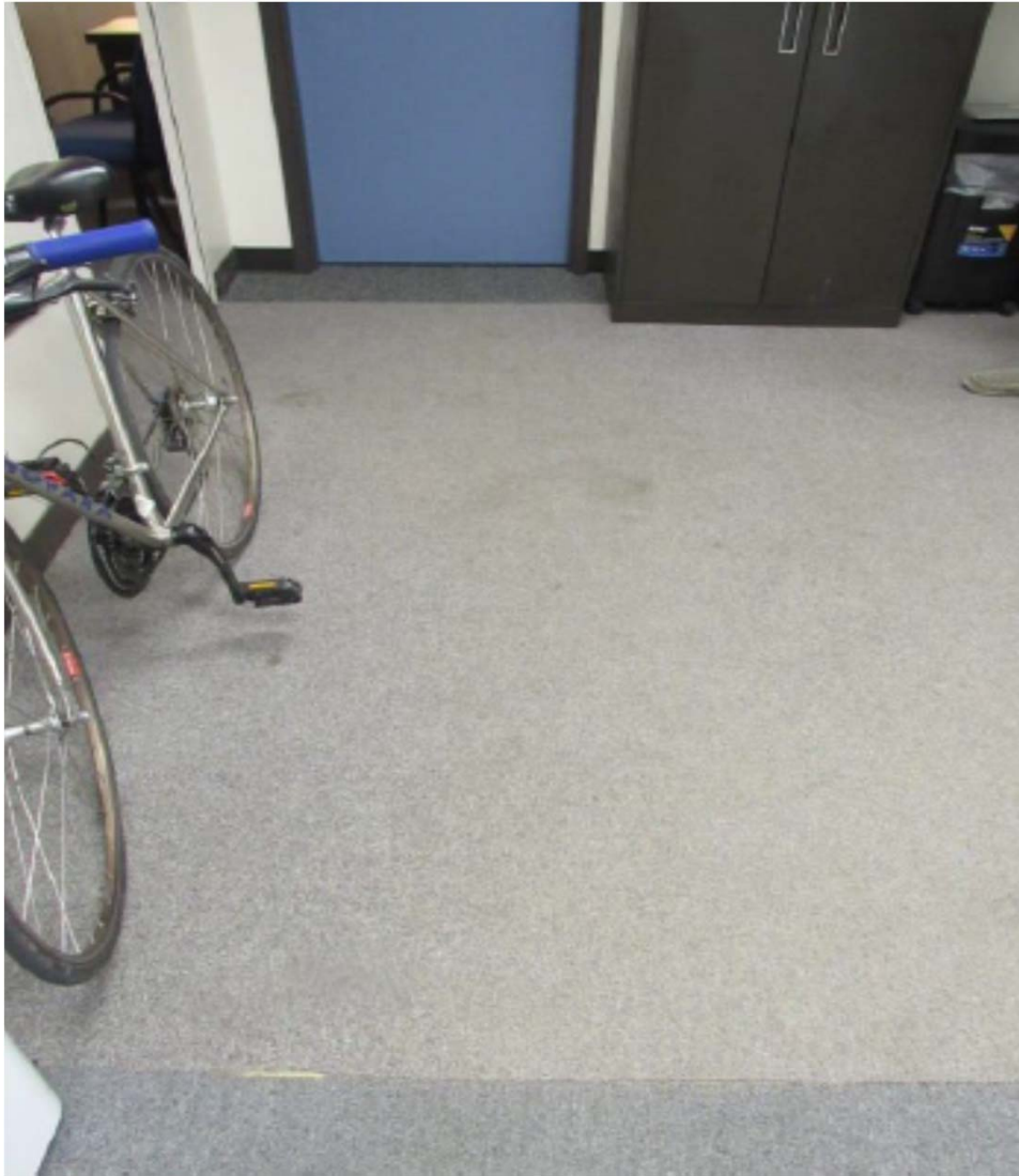
Image #1: Code Enforcement Office. Note the three different carpets used as a makeshift solution.
