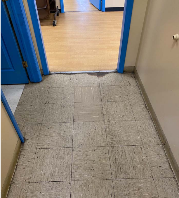
Images #7, 8 and 9: GWC Interior: Damaged Flooring
