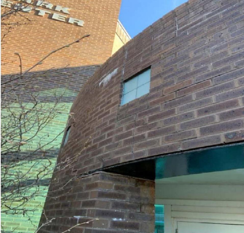
Image #5: Typical cracks in brick façade, with efflorescence.
