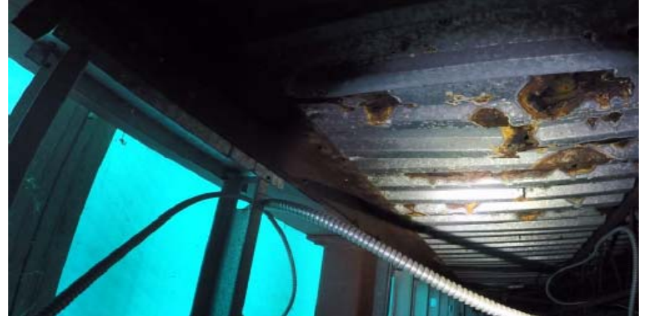
Image #2: Typical steel decking holes and buckling.
