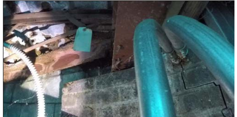
Image #4: Typical steel beam & joist and crack in brick. Note further corrosion and pitting at steel.
