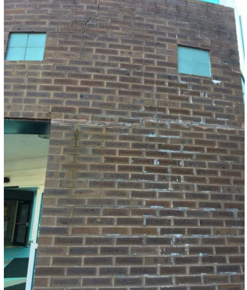
Image #6: Typical cracks in brick façade, with efflorescence.
