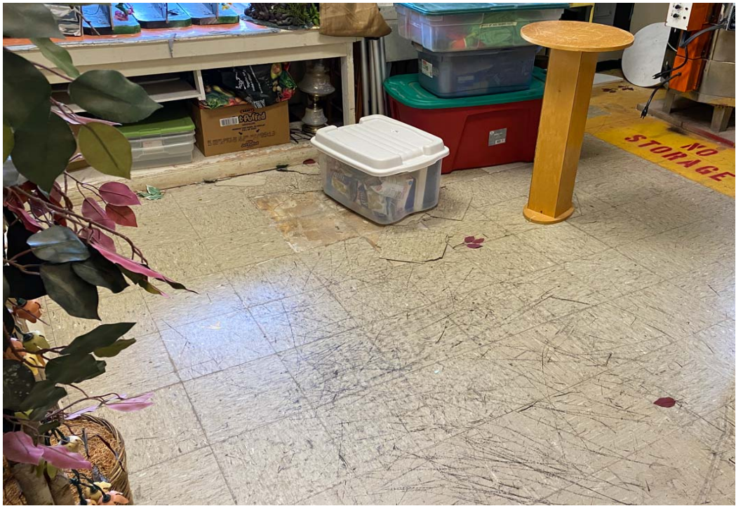
Images #10 and 11: GWC Interior: Damaged Flooring
