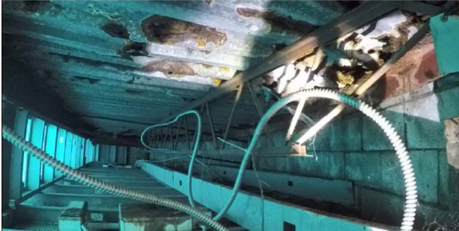
Image #1: Typical steel decking. Note corrosion and holes at decking.
