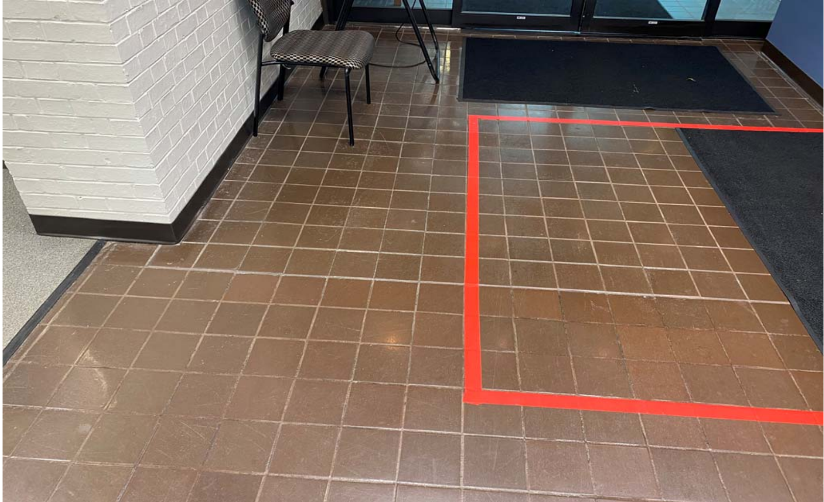
Image #13: City Hall lobby tiles. Note damage and cracks between/in tiles.
