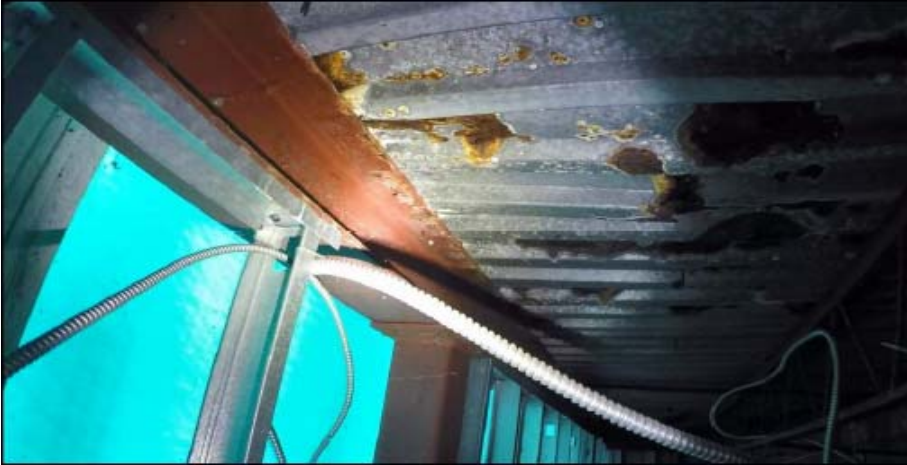
Image #3: Typical decking, studs, beam and column. Note corrosion, holes and buckling of decking.
