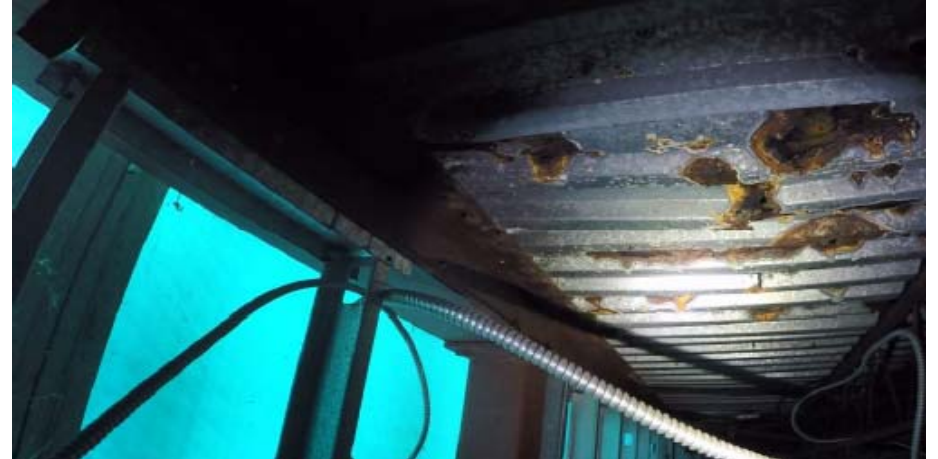
Image #2: Typical steel decking holes and buckling.
