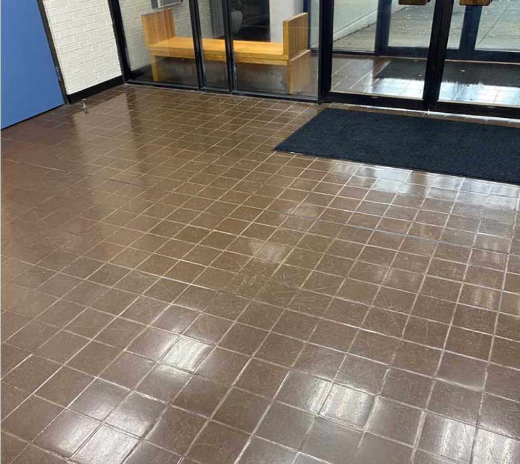
Images #11 and 12: City Hall lobby tiles. Note damage and cracks between/in tiles.
