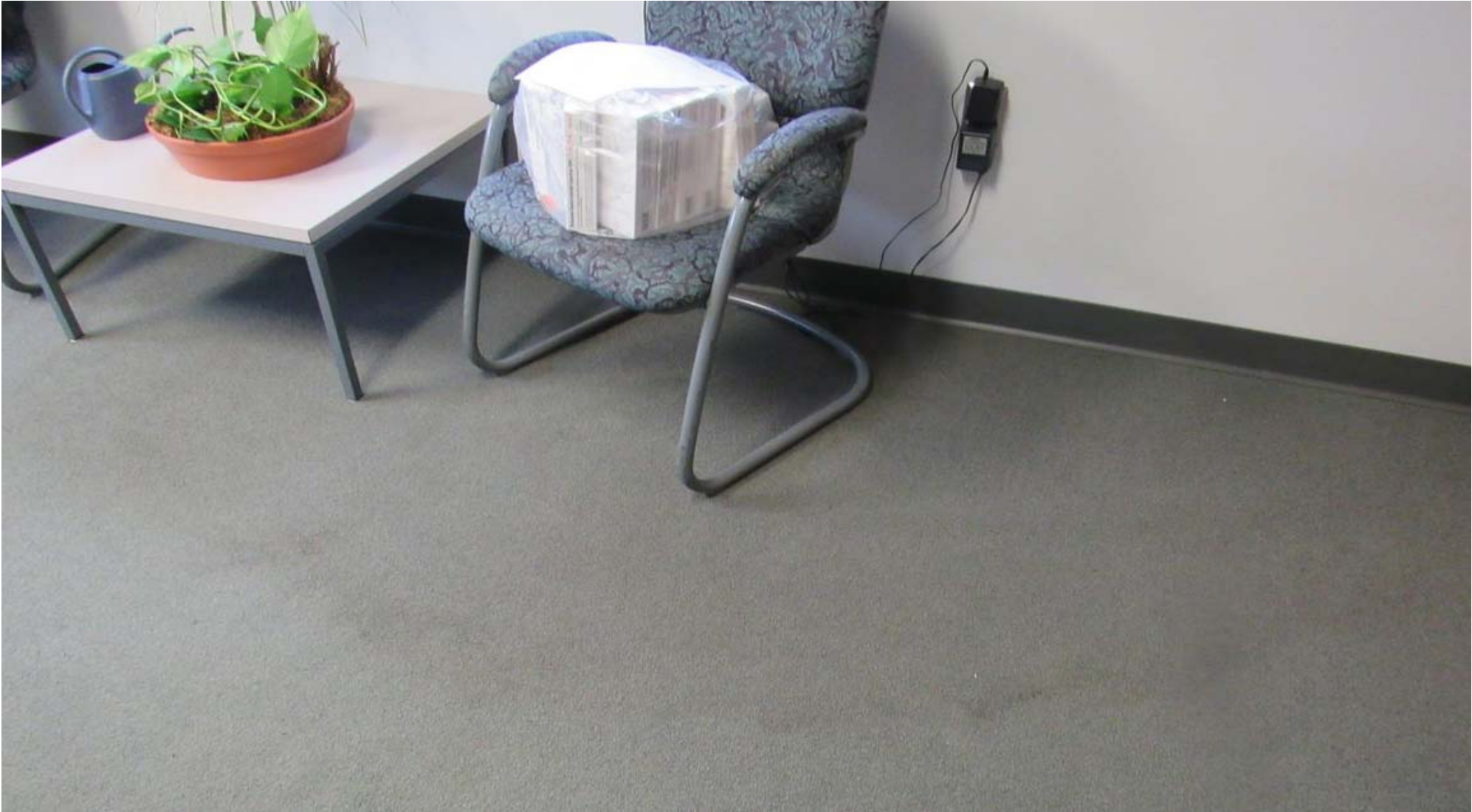
Image #5: Deputy Chief's office. Note water staining due to leaking roof and window (now fixed) over past several years.
