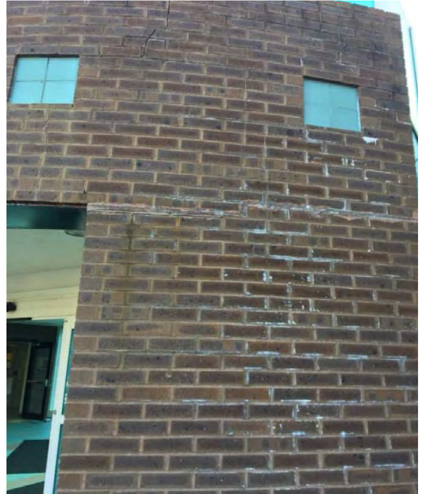
Image #4: Typical cracks in brick façade, with efflorescence (BEFORE).
