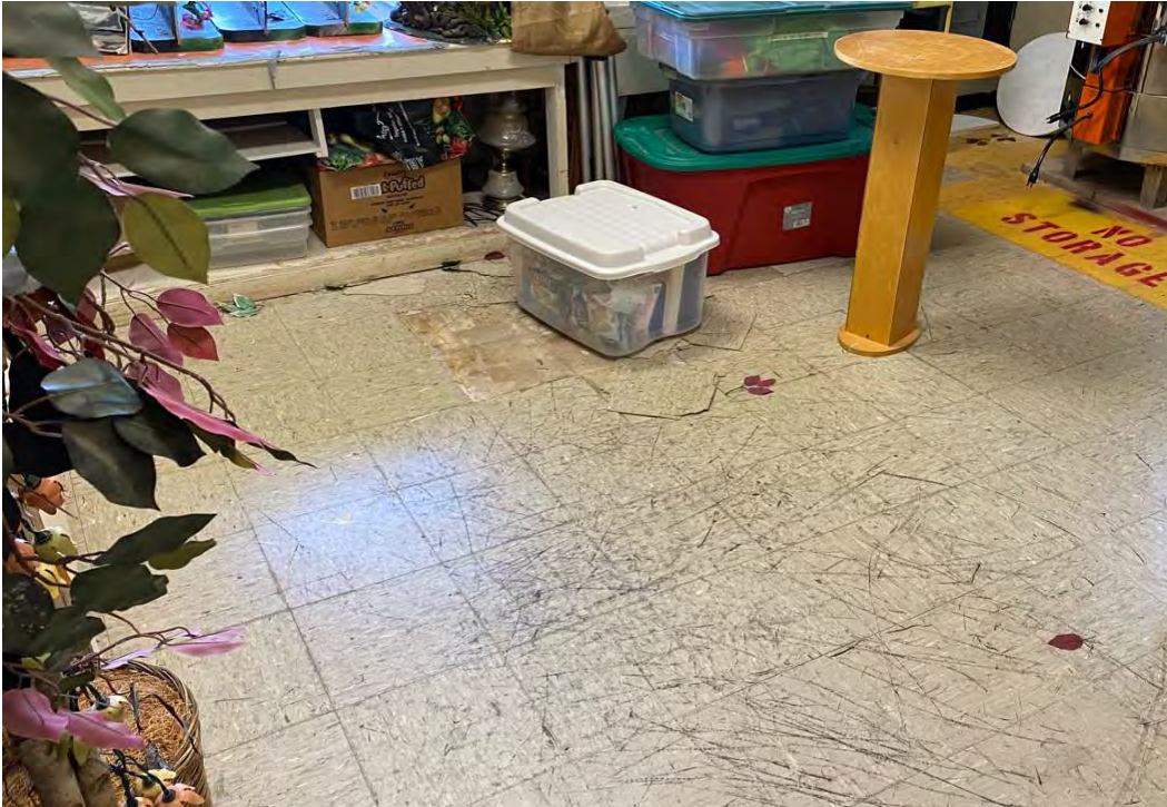
Images #10 and 11: GWC Interior: Damaged Flooring
