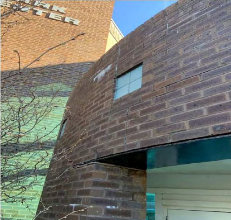
Image #3: Typical cracks in brick façade, with efflorescence (BEFORE).
