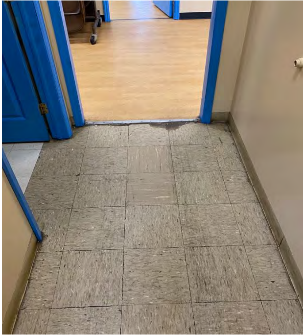
Images #7, 8 and 9: GWC Interior: Damaged Flooring
