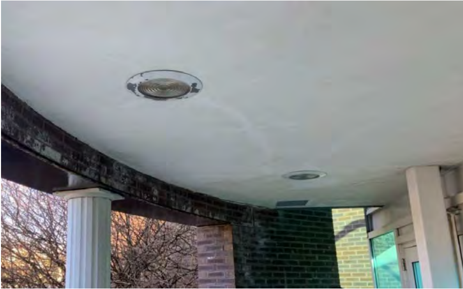
Image #1: Typical lentil and efflorescence in brick. Note condition of ceiling showing water damage (BEFORE).
