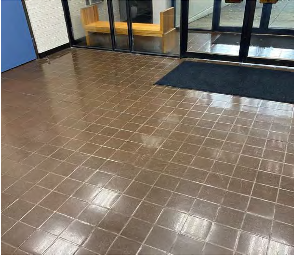
Images #5 and 6: City Hall lobby tiles. Note damage and cracks between/in tiles (BEFORE).
