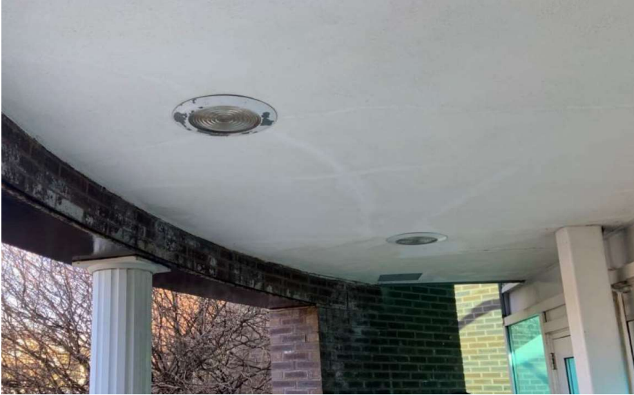
Image #1: Typical lintel and efflorescence in brick. Note condition of ceiling showing water damage (BEFORE).
