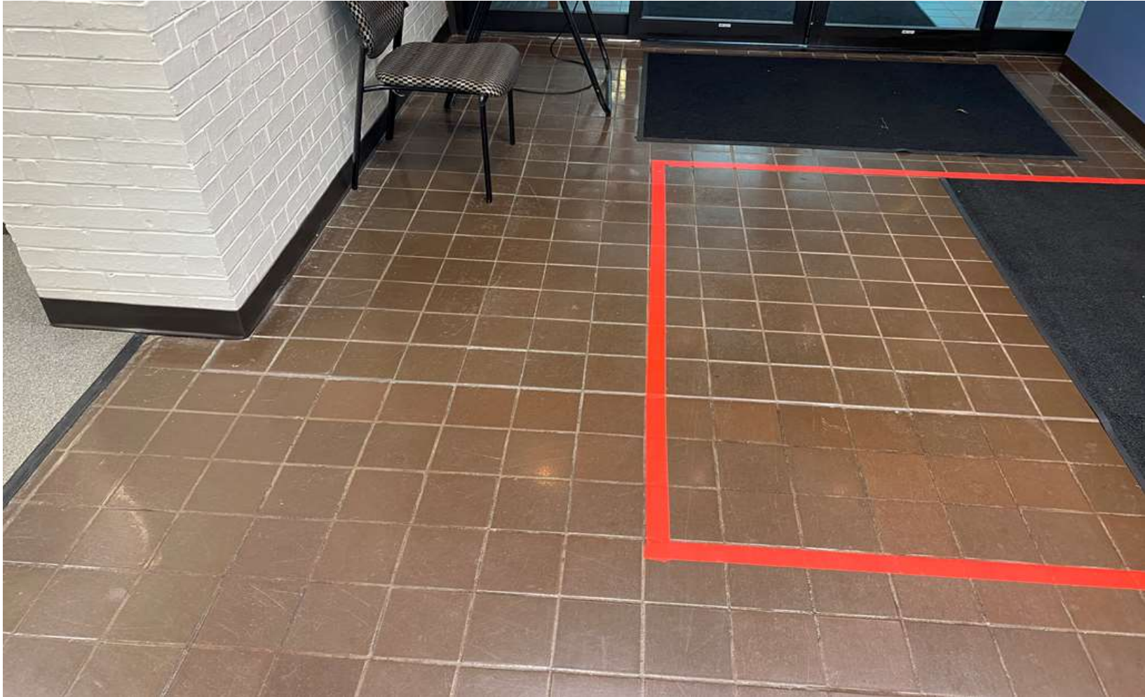
Image #7: City Hall lobby tiles. Note damage and cracks between/in tiles (BEFORE).
