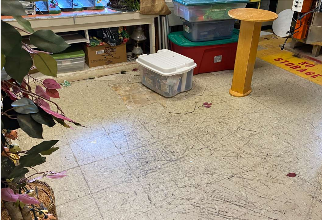
Images #10 and 11: GWC Interior: Damaged Flooring
