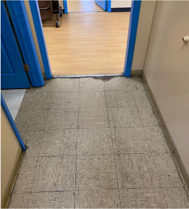
Images #7, 8 and 9: GWC Interior: Damaged Flooring
