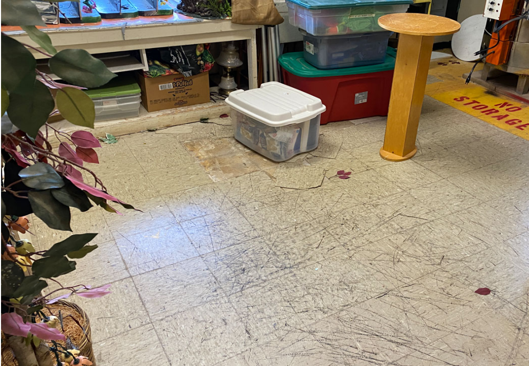
Images #10 and 11: GWC Interior: Damaged Flooring
