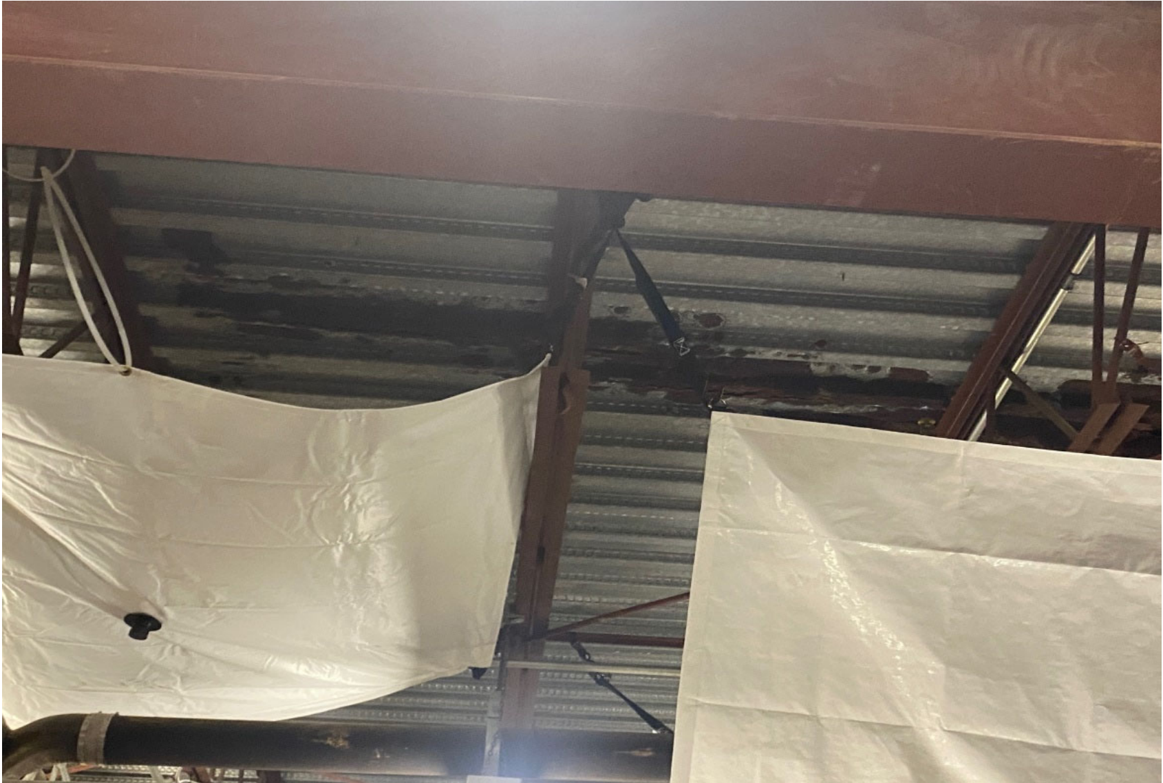
Image #3: Corrosion of metal decking under sally port
