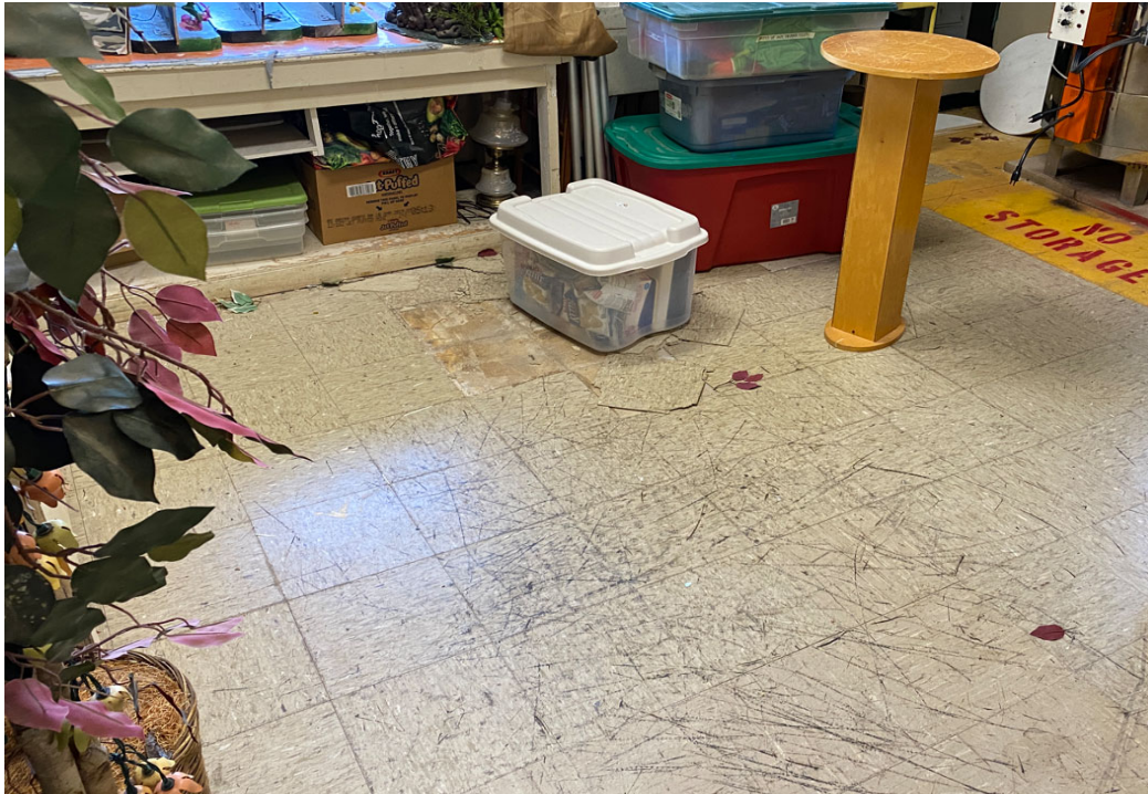
Images #10 and 11: GWC Interior: Damaged Flooring
