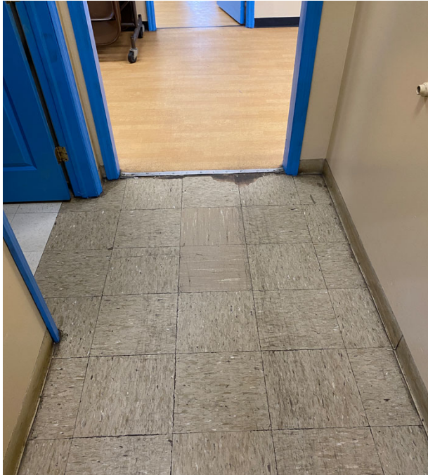
Images #7, 8 and 9: GWC Interior: Damaged Flooring
