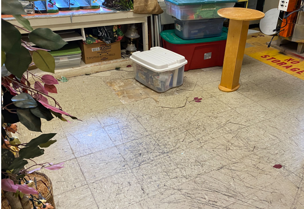
Images #10 and 11: GWC Interior: Damaged Flooring
