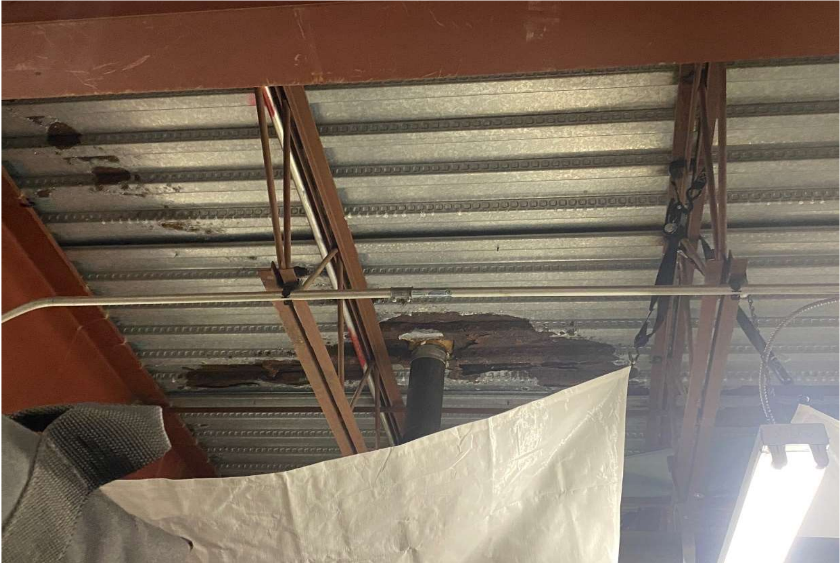
Image #5: Corrosion of metal decking under sally port
