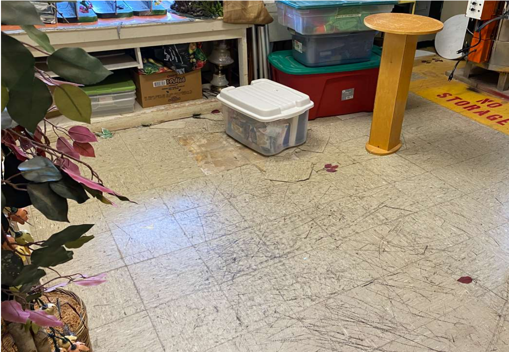
Images #10 and 11: GWC Interior: Damaged Flooring
