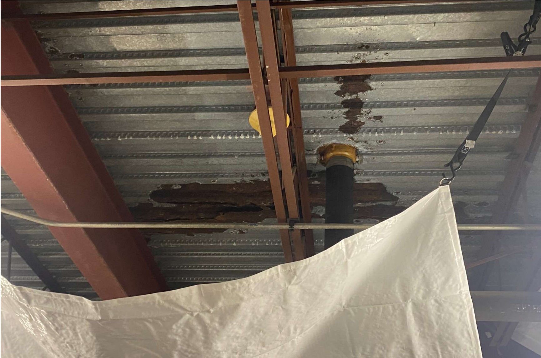
Image #4: Corrosion of metal decking under sally port
