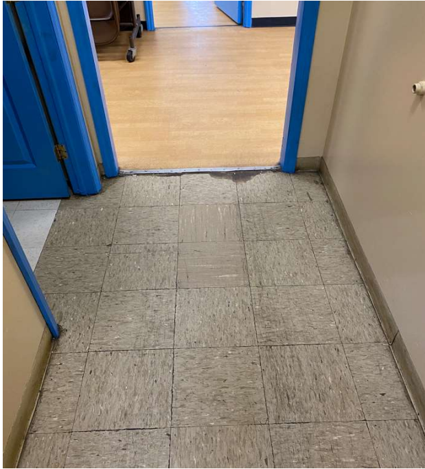
Images #7, 8 and 9: GWC Interior: Damaged Flooring
