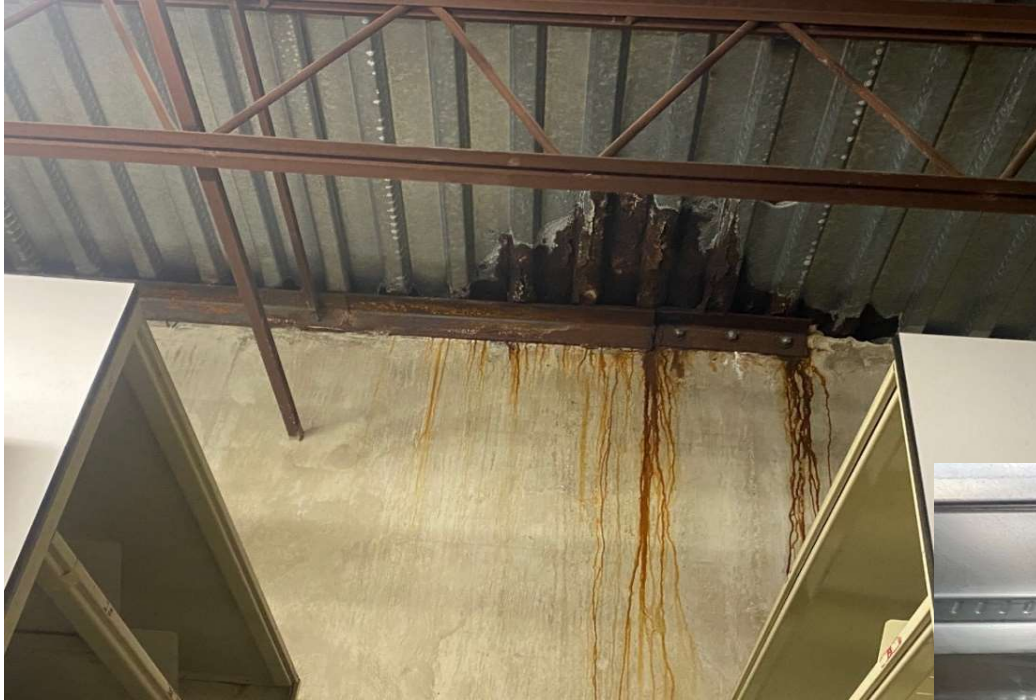
Images #6 & 7: Corrosion of decking along walkway between sally port and loading dock
