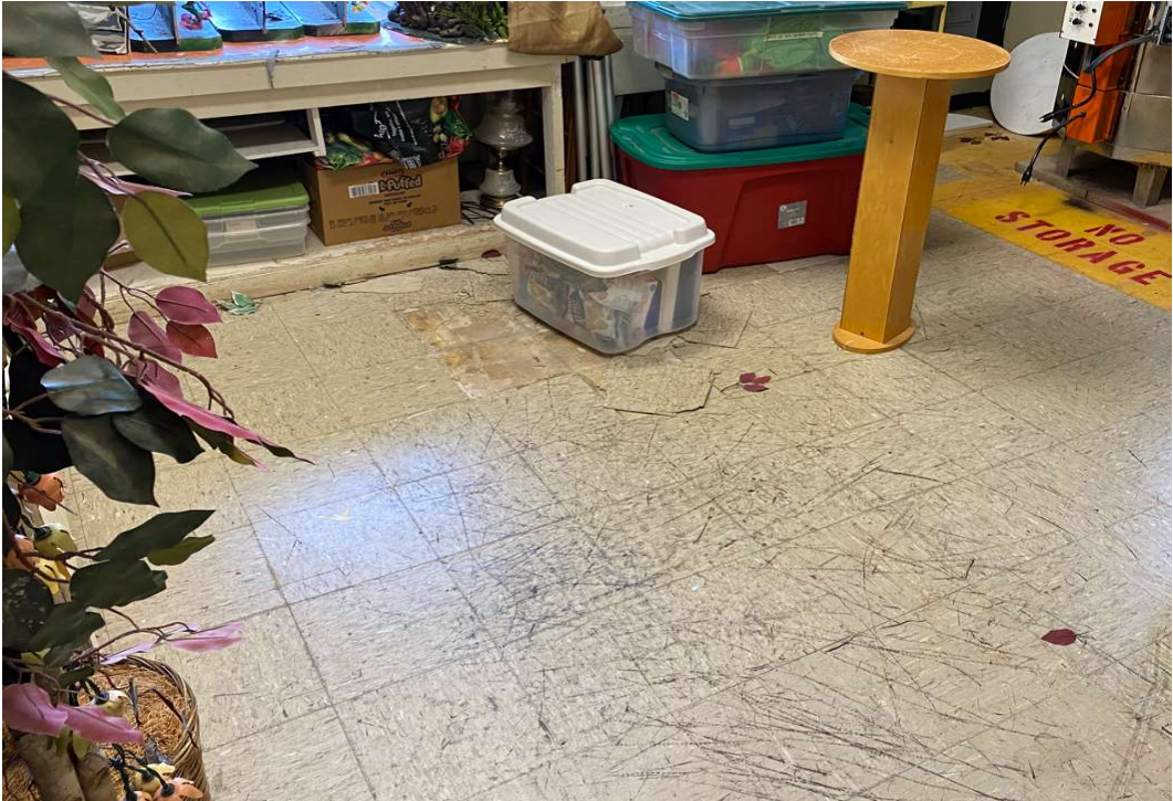
Images #10 and 11: GWC Interior: Damaged Flooring
