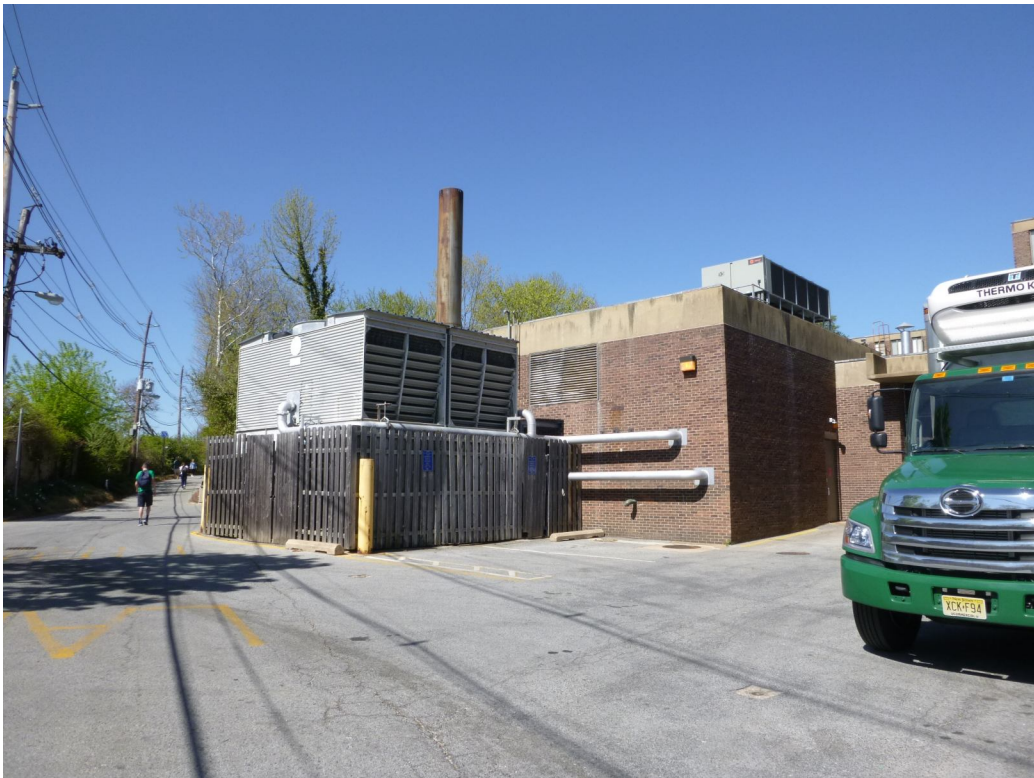
Photograph #2: Utility Plant located in the rear of the complex.
