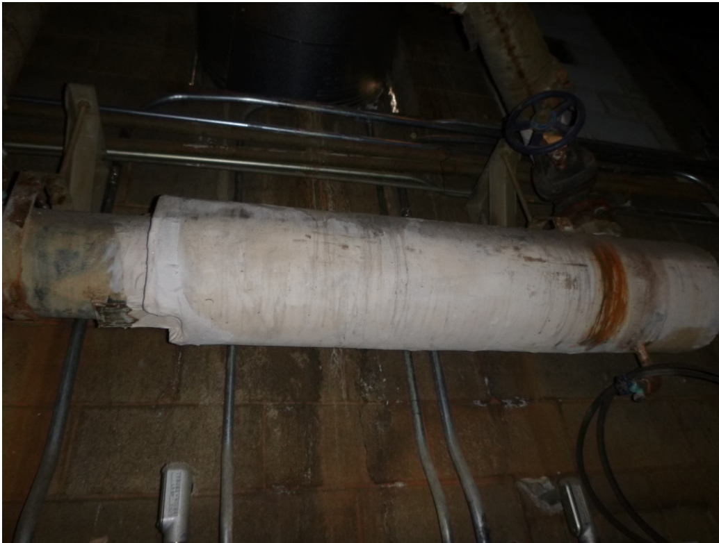
Photograph #7: Potential asbestos-containing pipe insulation in Utility Plant.
