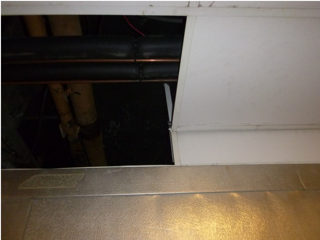
Photograph #8: Building overhead pipe chase with potential asbestos-containing materials.
